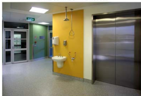
SAFETY STATION WITH SAFETY SHOWER, EYE WASH AND HAND BASIN AT THE ENTRANCE OF THE LAB
