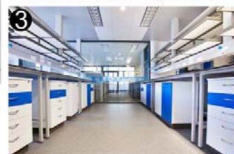
GAS, WATER AND POWER RETICULATED ON SERVICE DROPPERS. ALLOW TO FREE THE BENCH SPACE
