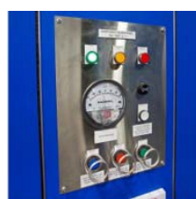
CENTRALISED ACCESS AND MONITORING POINTS
